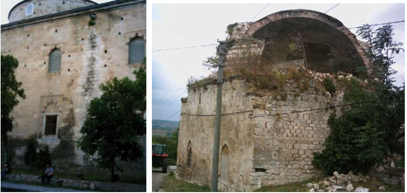
Figure 11. Eski Camii (Old Mosque) in Edirne was built of good quality limestone, but is being deteriorated by pollutants, sulfuric acid and carbon from domestic furnaces, which have combined with acid precipitation from long-range sources (left) and Şerbetdar Hasan Bey (Paşa) Camii at Vize province (Dal 2008).
