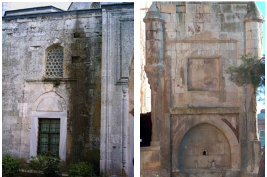
Figure 12. Acid precipitation attack the surface of the limestone and the reaction products run down the façade of II. Bayazıt Külliyesi (left) (Dal, 2005) and detail of the minaret of Old Mosque from Edirne: flaking and delamination are visible which cause material loss.
